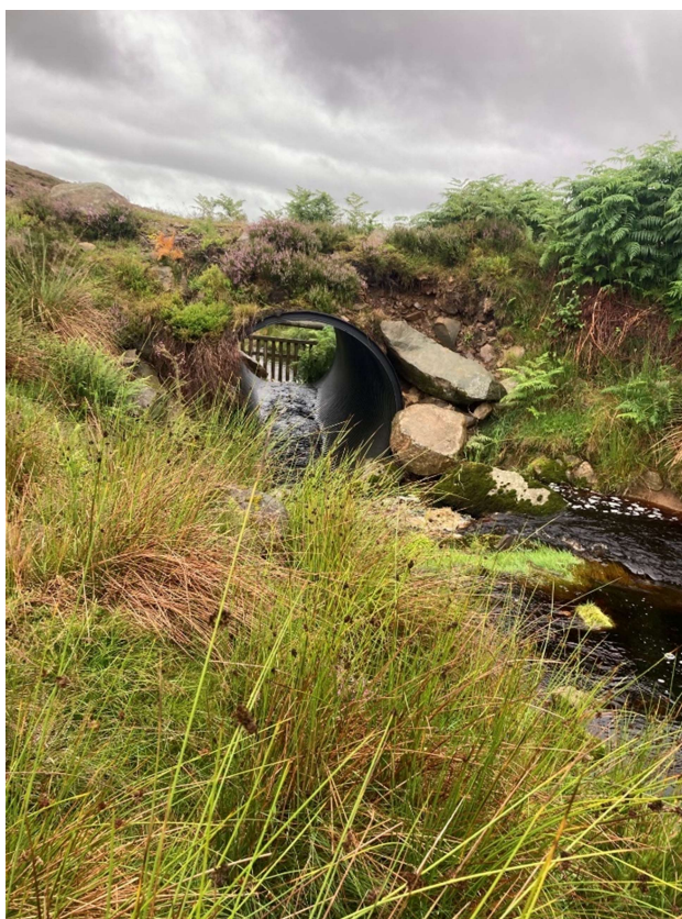
Photograph 3. T10 survey location: Culvert, potential barrier under certain flow conditions.
